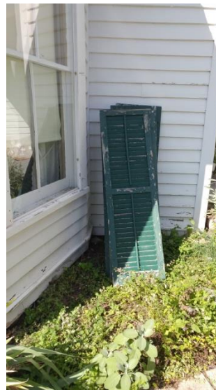
Summer 2017 Peeling Shutters
